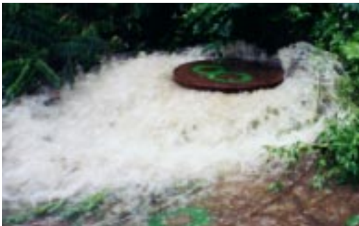
Overflowing manhole On Cover: A combined sewer overflow.
