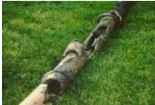
Broken house lateral line
